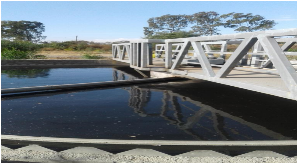
Figure:-6. Partial view of Secondary treatment plant- Reactor- Not functional, East African Tannery
