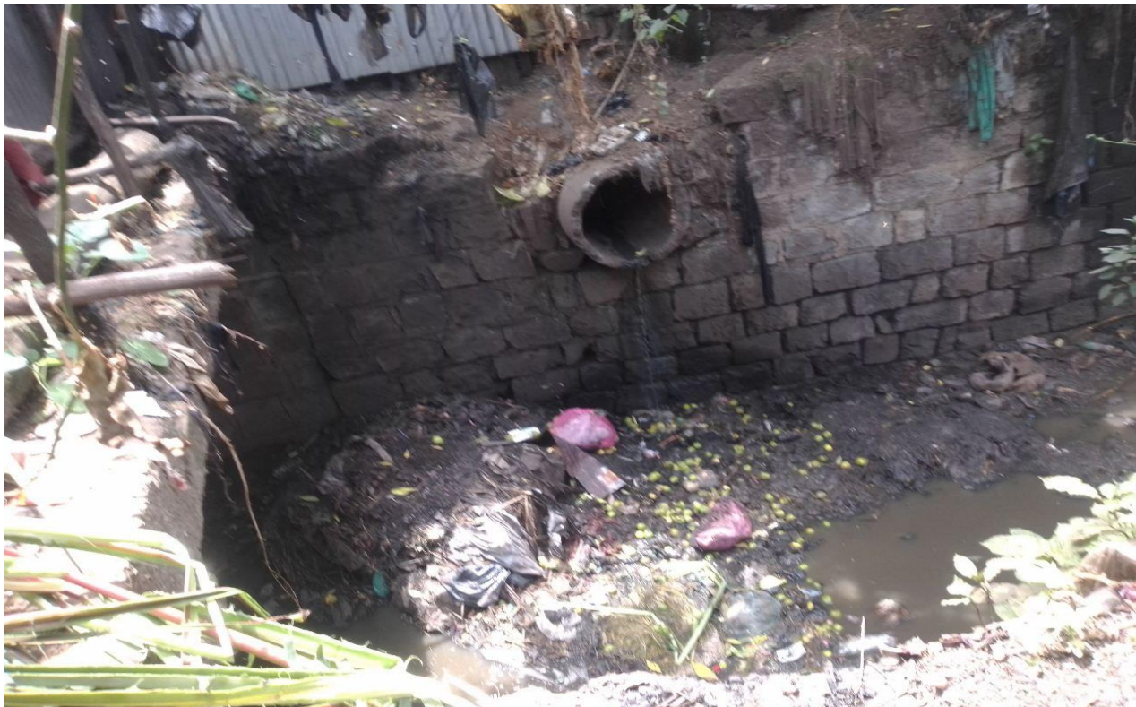
Figure 28. Toilet-connected drainage interring to the river
