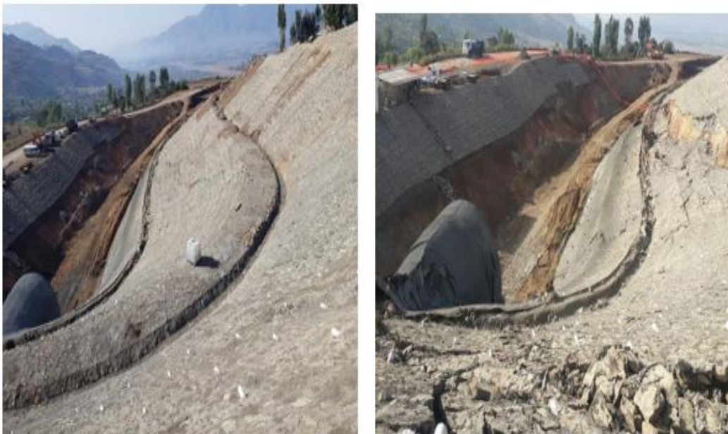
Figure 1. 1: (a) cracks developed tunnel portal slope (left) 1(b) tunnel portal failure(right)
