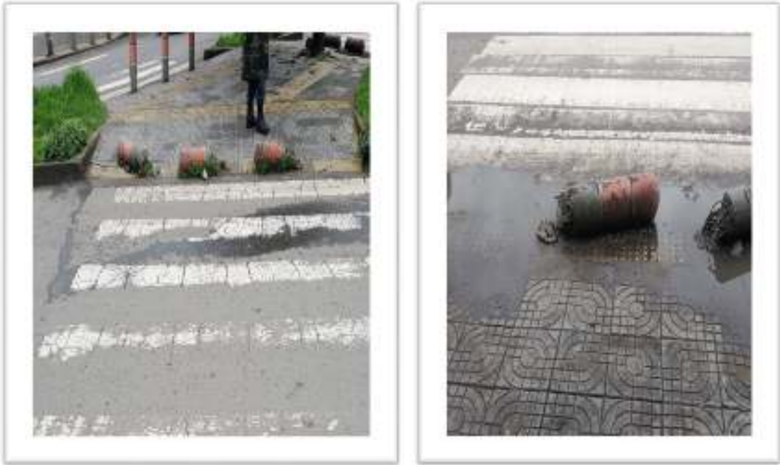
Picture 4.6.1.7 Blocked crossing with bollards needs maintenance in Ethio-China
