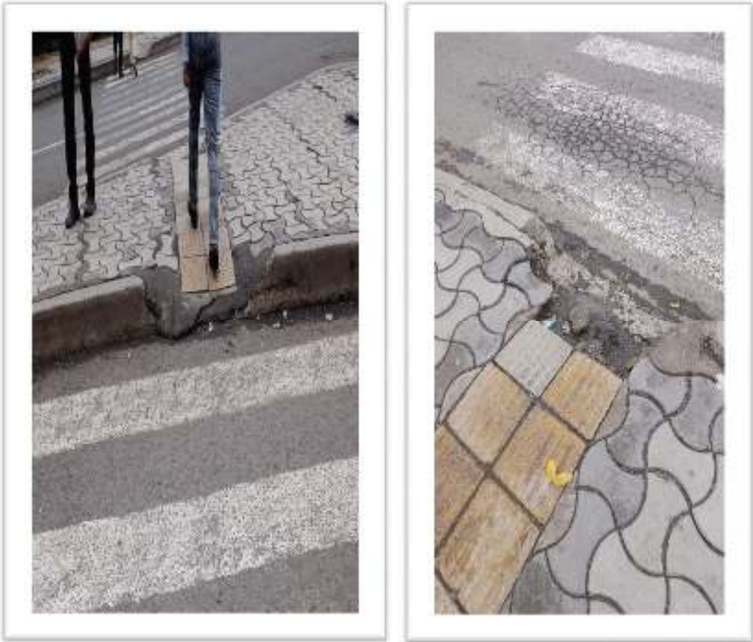
Picture 4.6.1.3 Medians (refuge islands) without proper ramp in Diaspora
