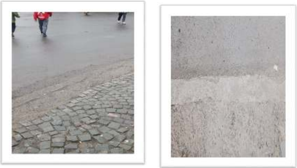
Picture 4.6.1.2 Uncomfortable curb ramp structure in Mikael
