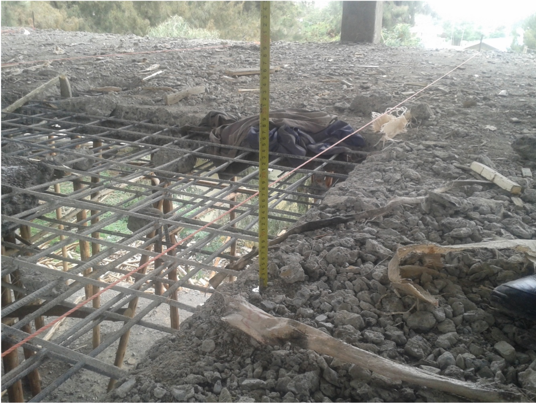
Figure 37 actual failure of slab by deflection
