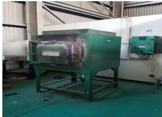
Figure 3.23 Heat treatment metal furnace machine
