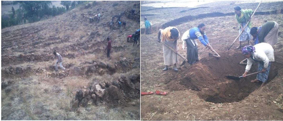
Fig.4.4 Stone bunds (left) and soil bunds (right) constructed by community participation, Source: WARDO 2015.
