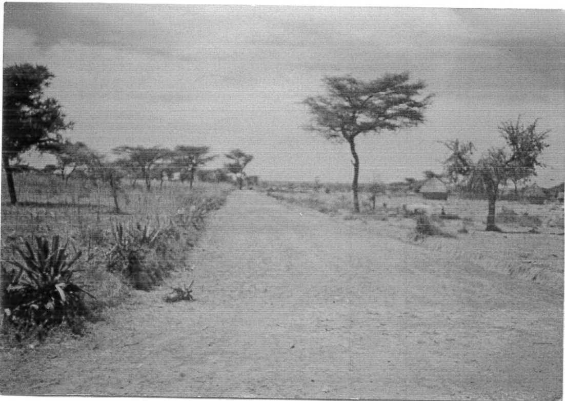
Figure 5: Road constructed or maintained in Chetu Getu in 2006 by PSNP Public work participants
