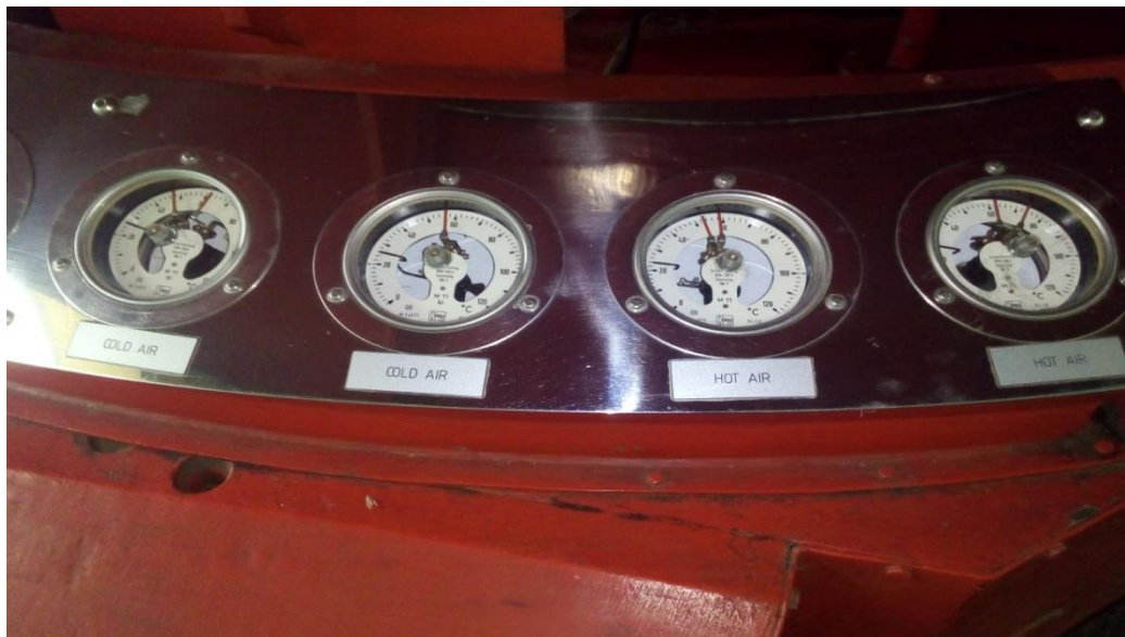
Fig.3.4 Temperature Measurement of Generator Cooling System
