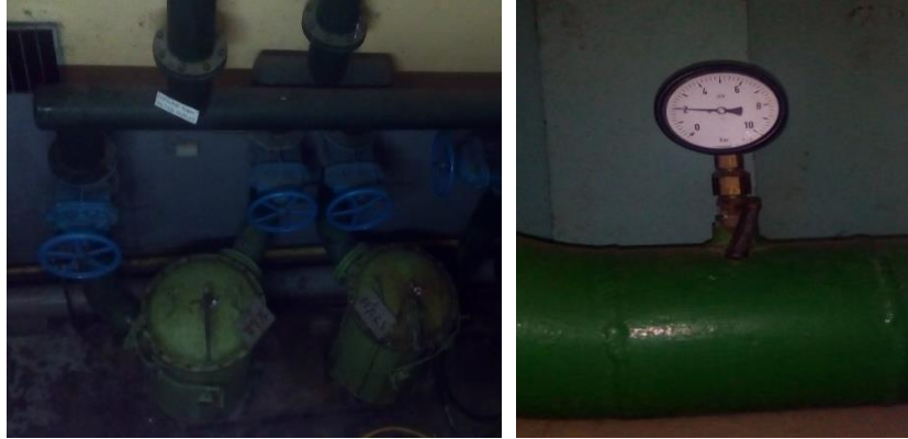
Fig.3.3 Cooling Water Filters and Their Pressure Gauge
