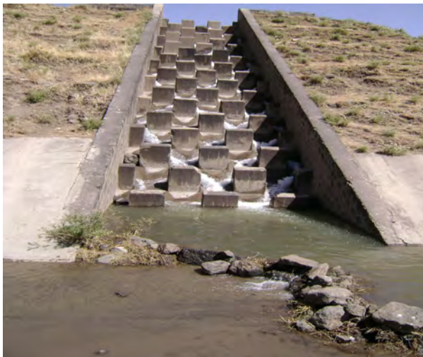
Fig. 2. Channel through which Mojar River was Diverted into the lake in December, 2008.
