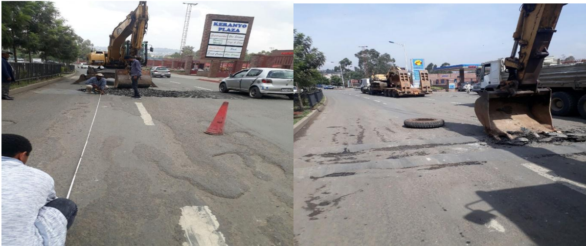
Figure 13: Torhayiloch –Mendida pavement condition measurement [2]
