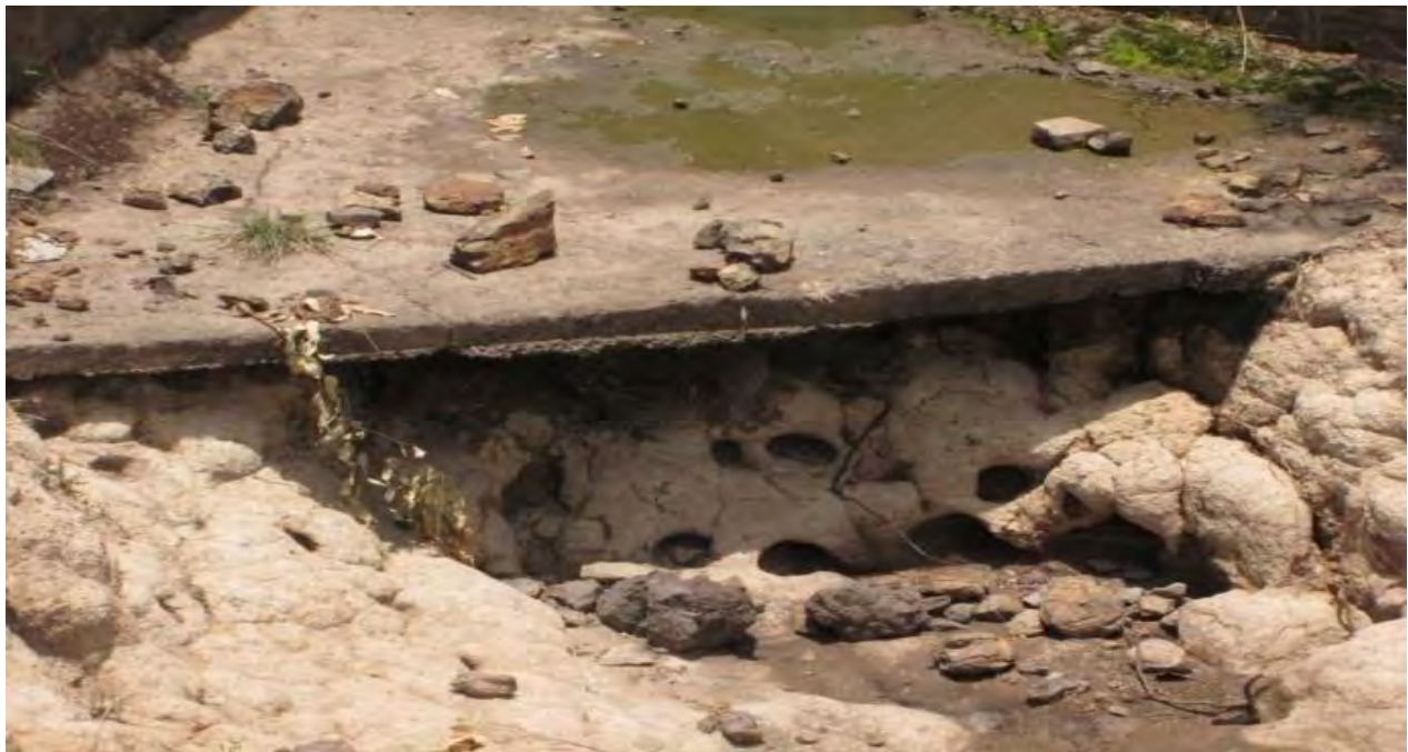
Figure 3.6a Cracking and scouring of paved water way
