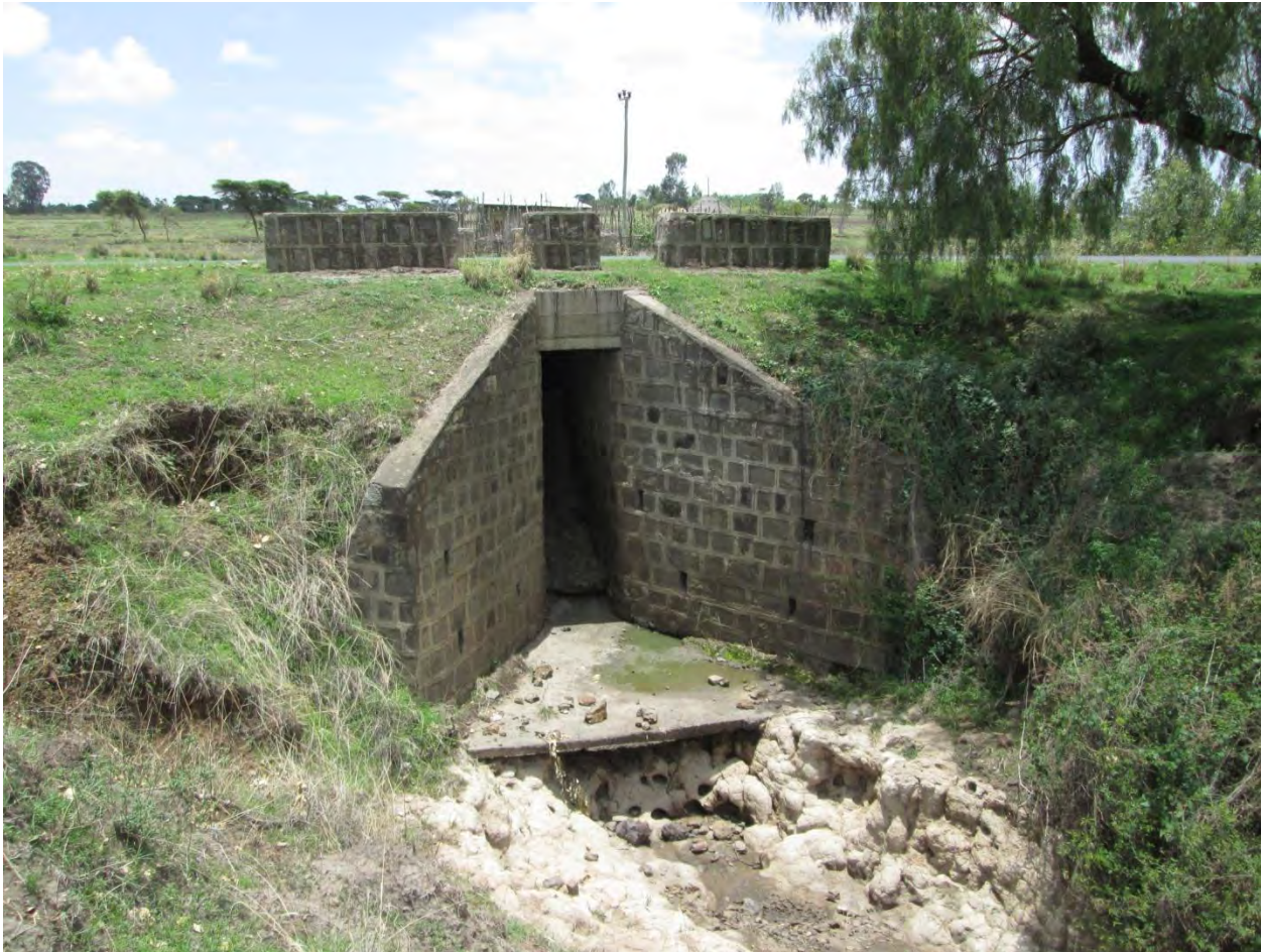
Figure 3.7b scouring of waterway outlet side
