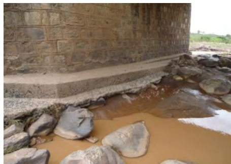
Figure 3.6:- Previous damage RC Slab culvert type Bridge
