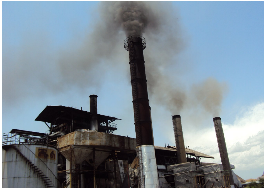
FIGURE 4.1-3: The Four Boilers' Chimney at MSF 7
