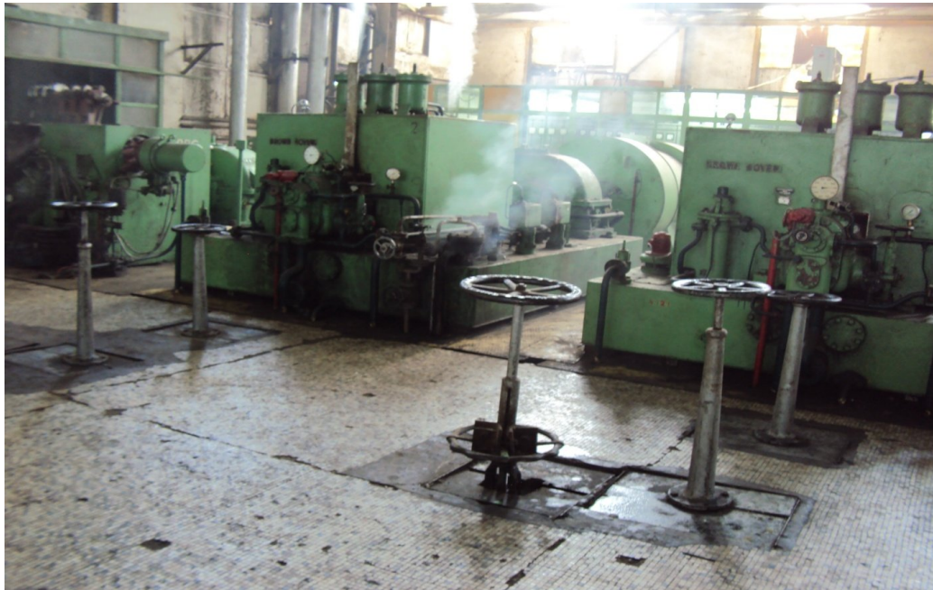
FIGURE 4.1-5: Partial View of the Three Turbo-alternators (Power Turbines) 9
