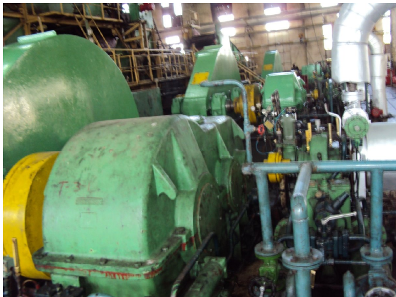
FIGURE 4.1-6: The Three Mill Turbines for Tandem A 10
