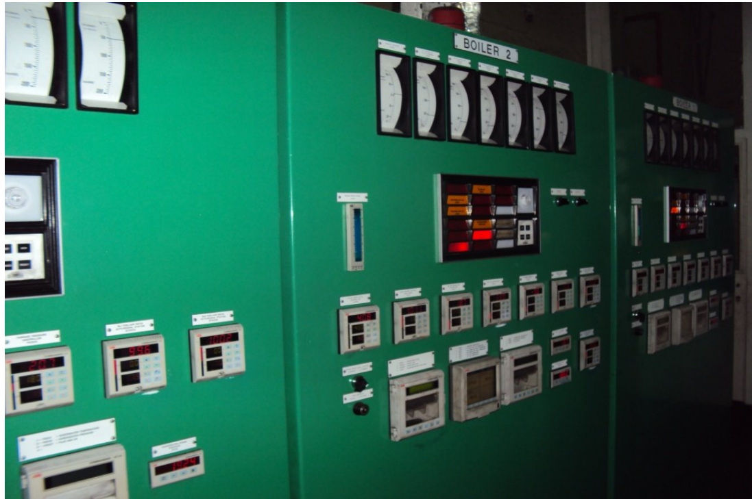
FIGURE 4.1-4: The Boilers' Control Panel at MSF 8
