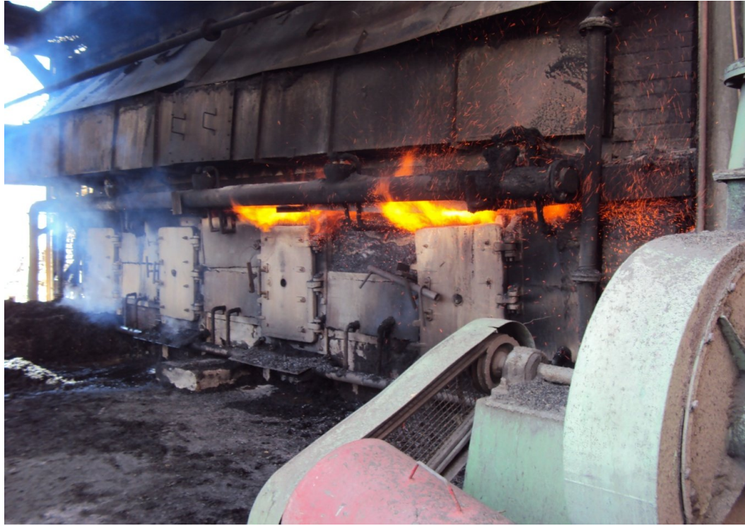
FIGURE 4.1-13: Typical Loss Area in one of the Furnaces 14
