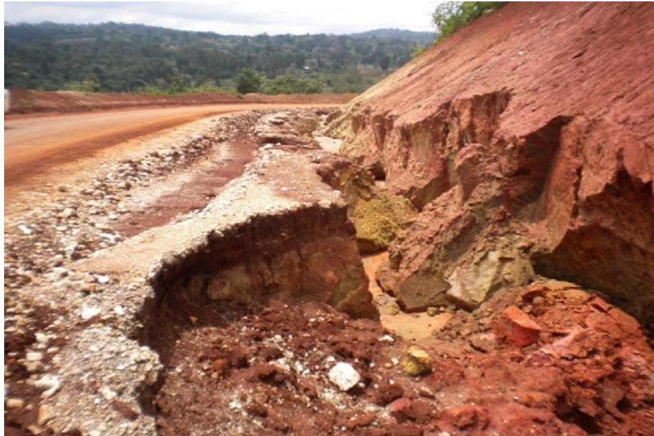
Plate. 4.1 Severe erosion in the rolling terrain (km 155+850, RHS), Photo, August, 2010
