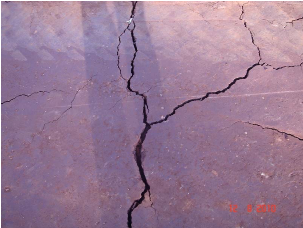
Plate 5.1 Cracks in clay due to drying (km156 + 900),
