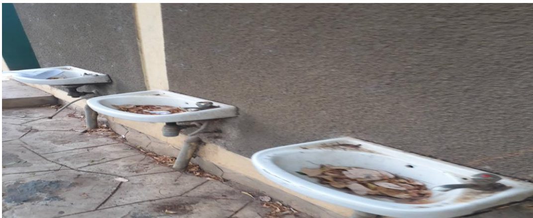
Gambella town secondary and prep students' toilet
