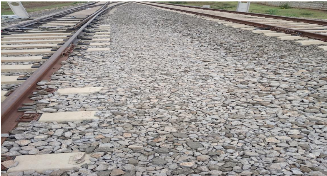
Figure 5. New ballast different from the designed standard (grading, strength) around Bishoftu
