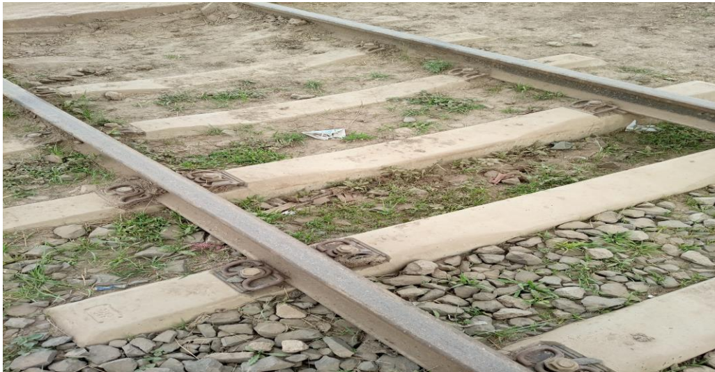
Figure 6. Fouled ballast around level crossing (Furi)
