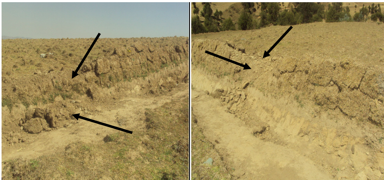
Figure 16: Fractured water way around Ya'i Chebo kebele.
