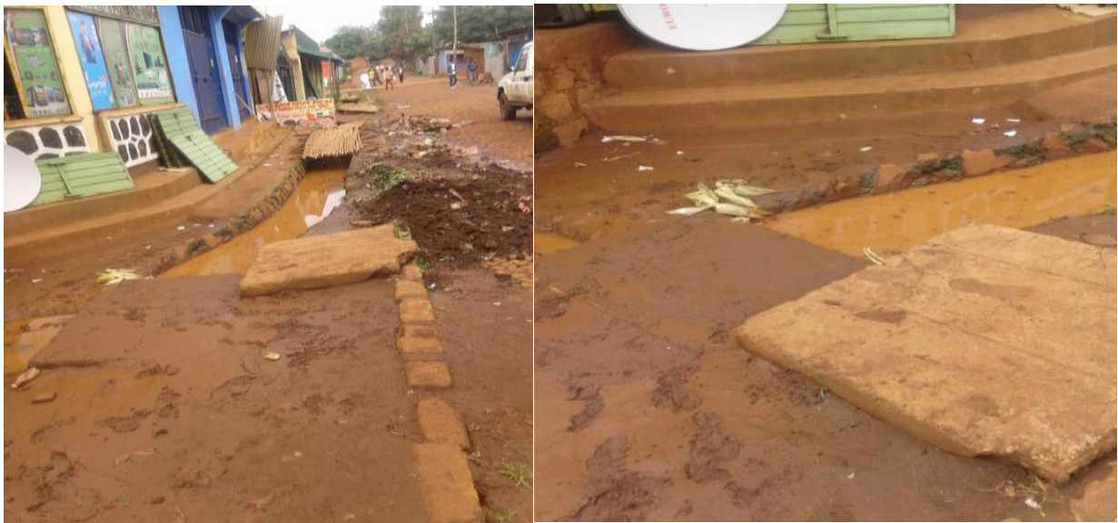
Figure 2.4: Rectangular open drains with poor outlet (July, 2018)
