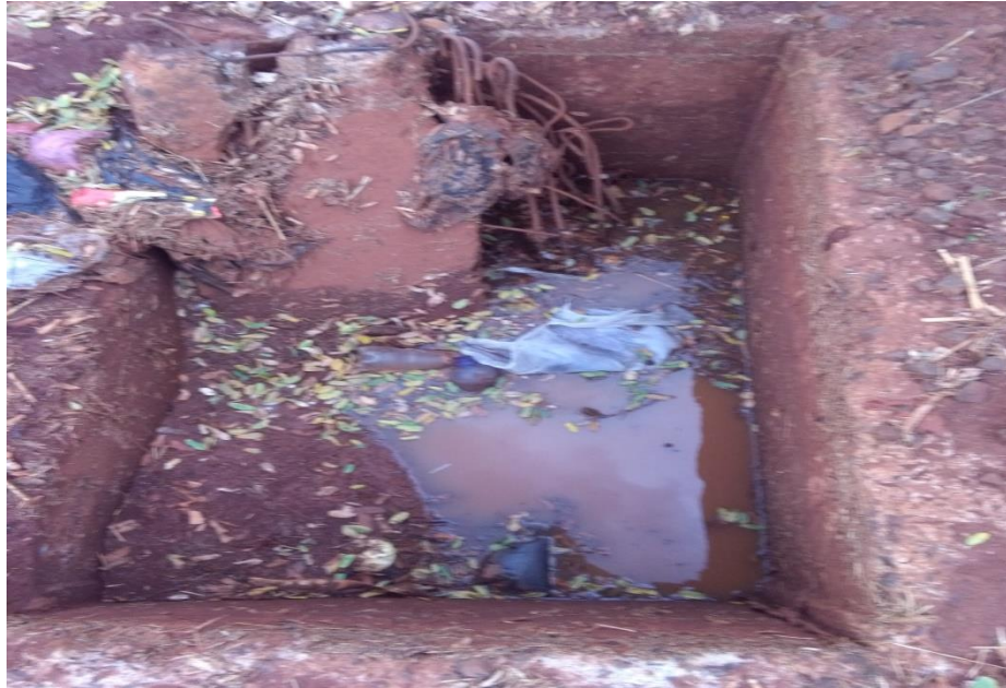
Figure 2.6: Failed drainage manhole (July, 2018)
