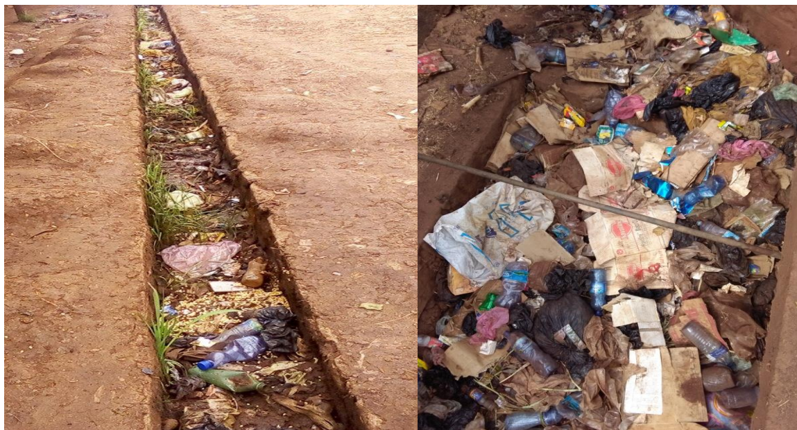
Figure 2.5: Excess sediment and dumping of solid waste in to drainage system (July, 2018)
