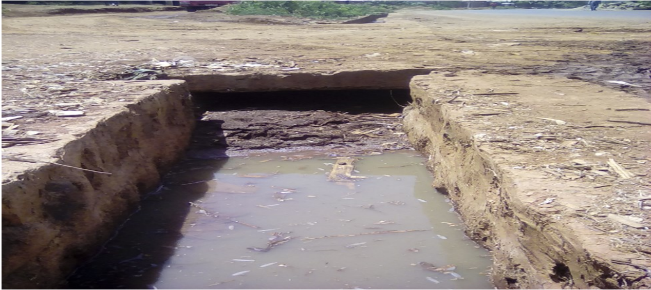
Figure 9 photographs of Junction 12 affected by sedimentation
