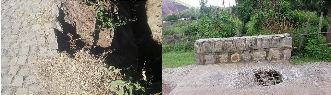
Figure 18. Poorly Constructed Drainage Lines (Source: Field Photograph, 2017)
