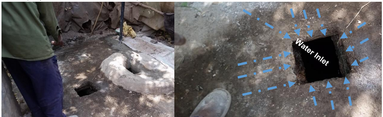
Figure 59. 2m by 3m Width with 4m Depth Hole for Flood Water Trapping (Source: Field Photograph, 2017)
