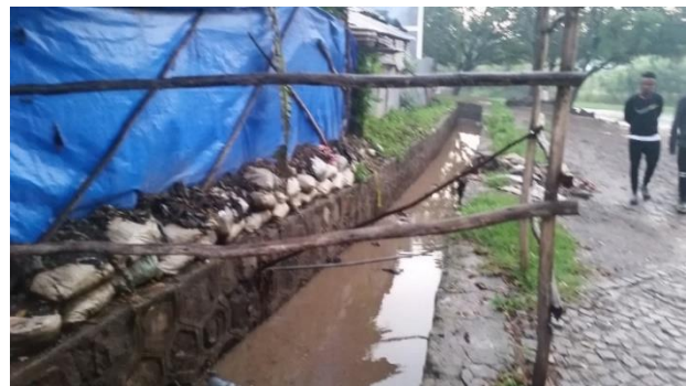
Figure 54. Sand Bags used as Blockage to Minimize the Water from Entering
