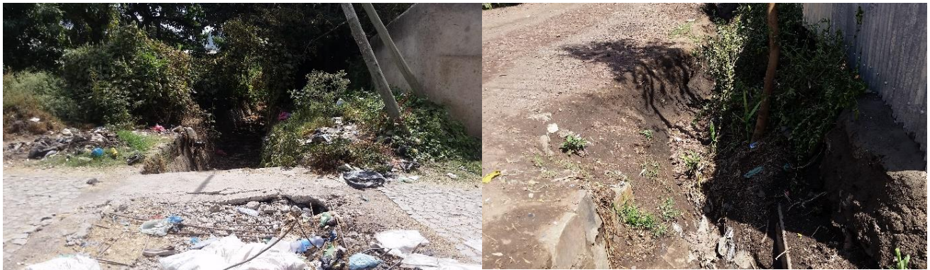
Figure 41. Deteriorating Drainage Lines (Source: Field Photograph, 2017 )
