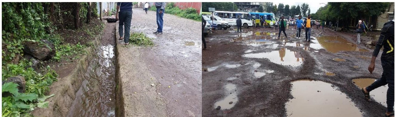
Figure 25. Deterioration of physical infrastructure
