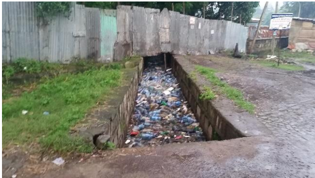
Figure 20. Clogged Drainage with Garbage (Source: Field Photograph, 2017)
