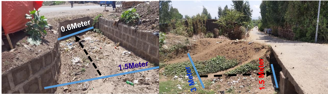
Figure 16. Incompatible drainage line Connection
