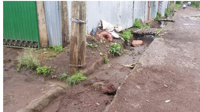
Figure 19. Sedimentation of Soil in the Drainage
