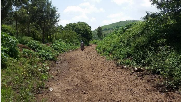
Figure 38. Non-Paved Drainage line serving as Walkway during Dry Season
