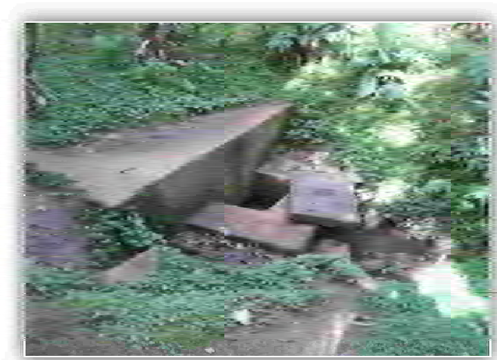
Figure 5.17 Non functional spring cap and failed spring box in Ezo Otte
