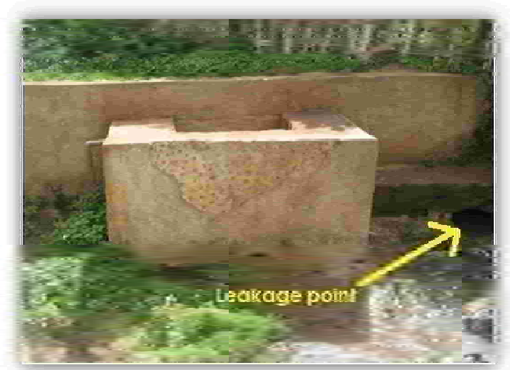
Figure 5.16 Completely failed spring cap in Doko Shaye keble
