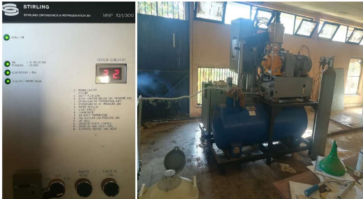
Figure 20. Liquid nitrogen plant in Bahir Dar town, Amhara region
