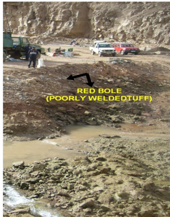
Plate 4.2 Red bole at the river bed channel section of the dam foundation
