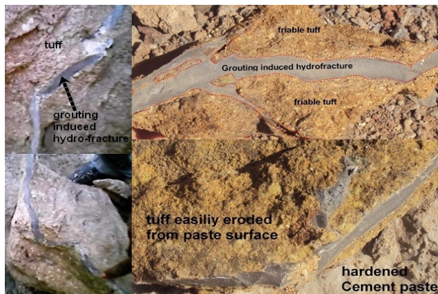
Plate 6.1 Grouting induced hydro-fracturing on tuff (left abutment)
