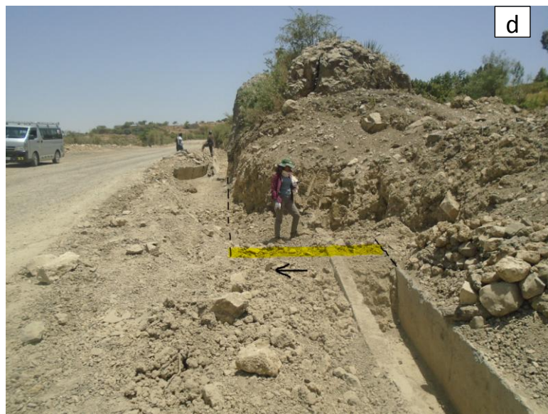
Figure 3-9 Current state of the landslide in the area (Kurur Village along main Asphalt road from Gohastion to Dejen, at 28 Km from Gohastion. (a) boulders of basaltic rock in the colluvium (b) and (c) head scarpments and cracks observed on site (d) recent slide at around 11 Km from Gohastion in the Gorge along the same highway.
