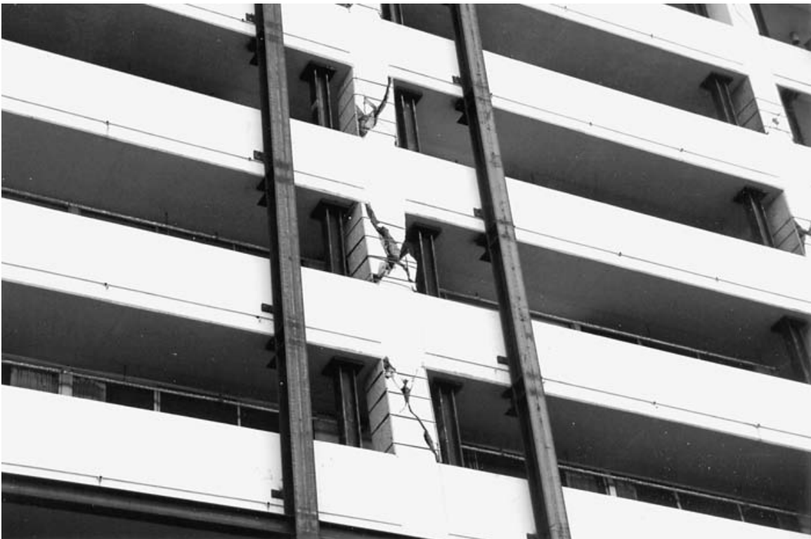
Figure 1-3 Reinforced-concrete columns severely damaged in the Northridge earthquake, Champagne Towers, Santa Monica, CA.
