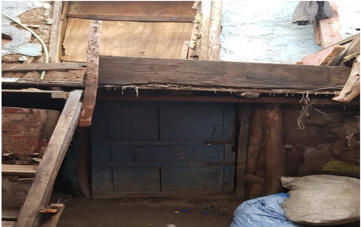
Figure 5: Housing condition of wereda seven
