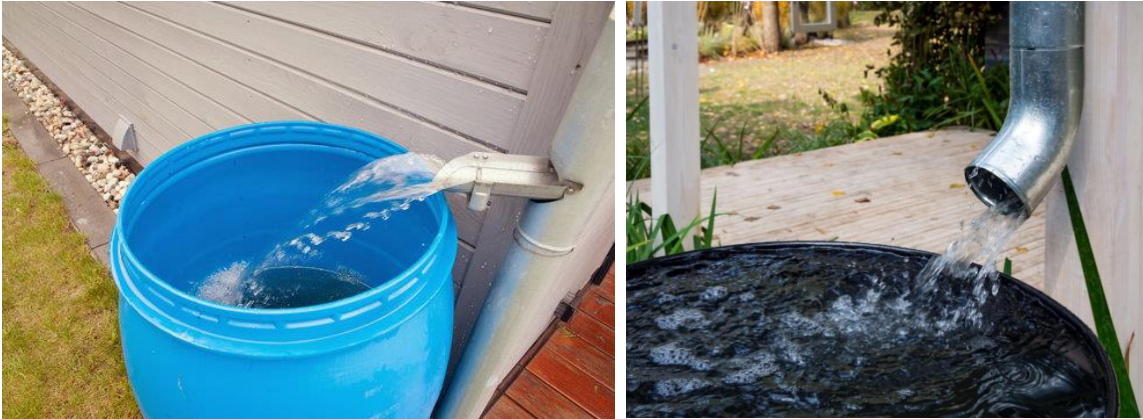
Figure 0.16: Rainwater harvesting during the rainy season (open source)
