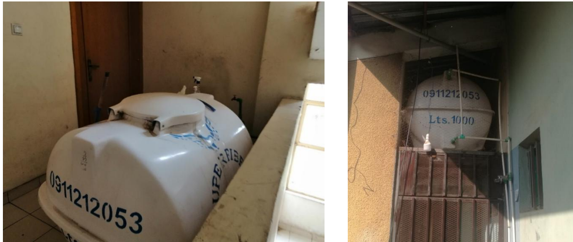
Figure 0.18: Elevated water tanker (own survey)
