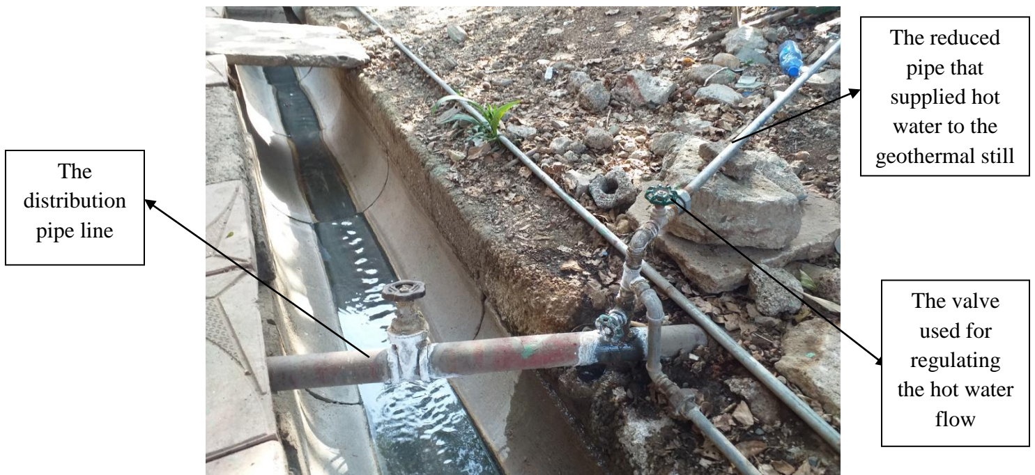
Figure 3. 17: The reduced hot water from the distribution pipe line
