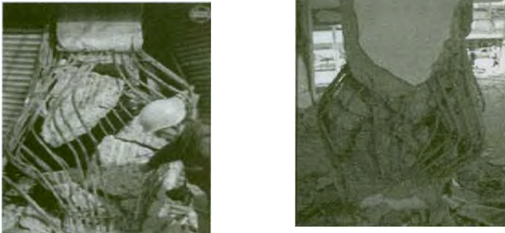
Figure 1.1 Failures due to Lack of Confinement [8]
