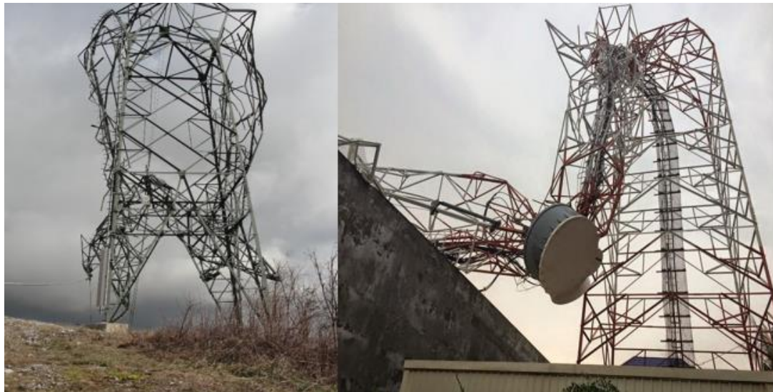
Figure 7: Self-supporting Communication tower failure
