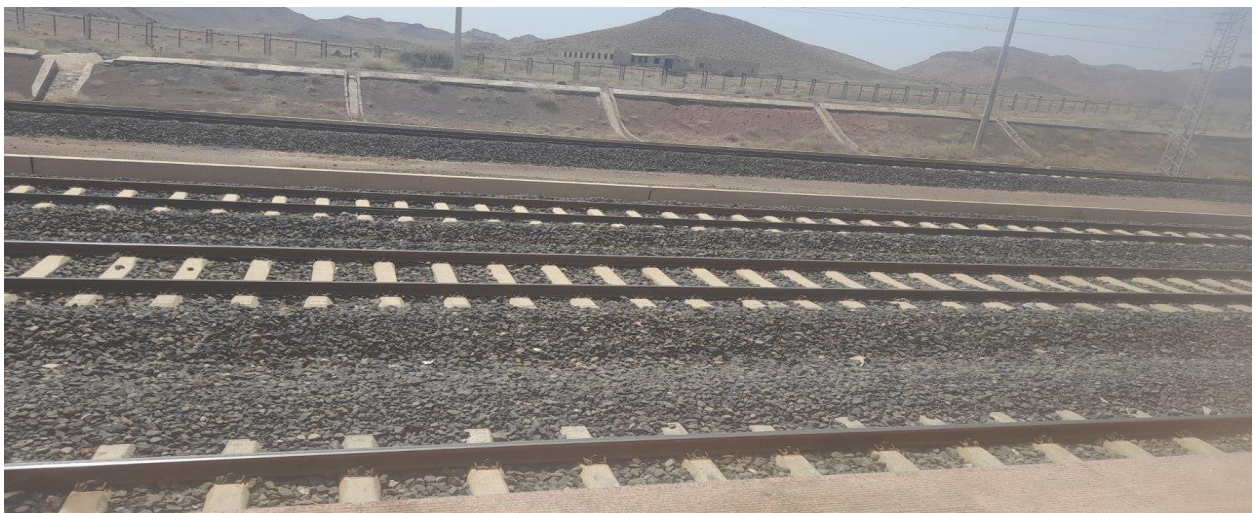
Figure 13: Surface fines and high degraded ballast at K663+500 (Dewele)
