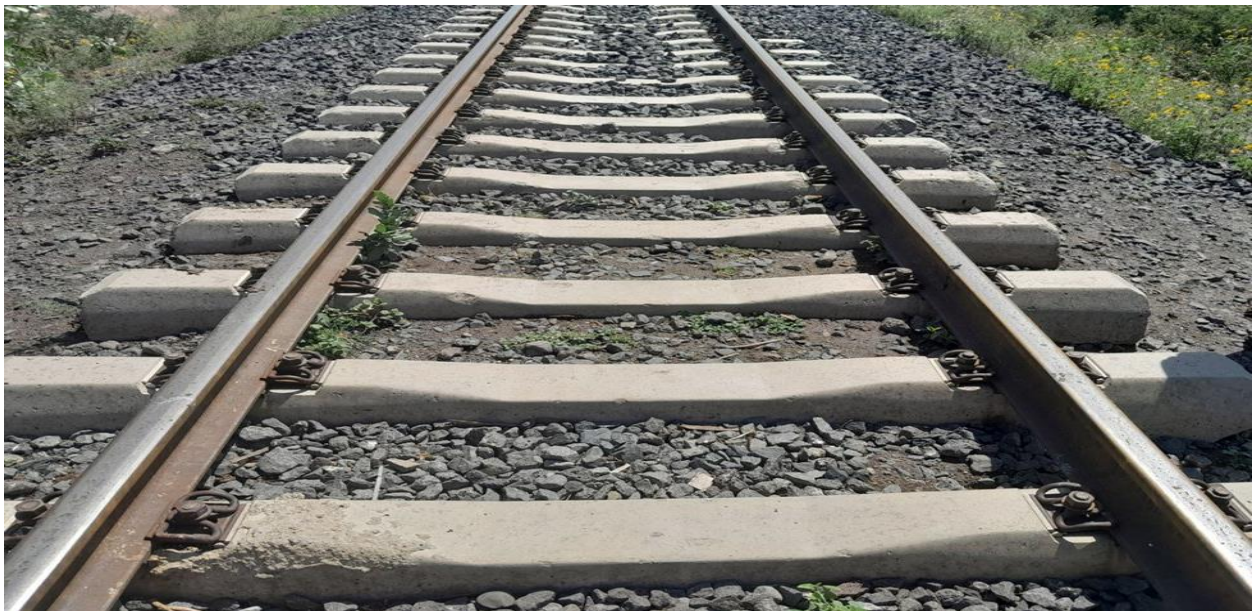
Figure 10: Missing crib and shoulder ballast and vegetation at K392+100 (Bike)
