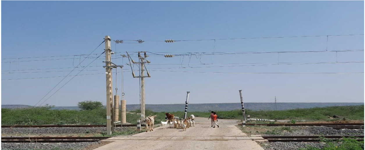
Figure 11: Fouled ballast around level crossing at K459+200 (Dire Dawa)
