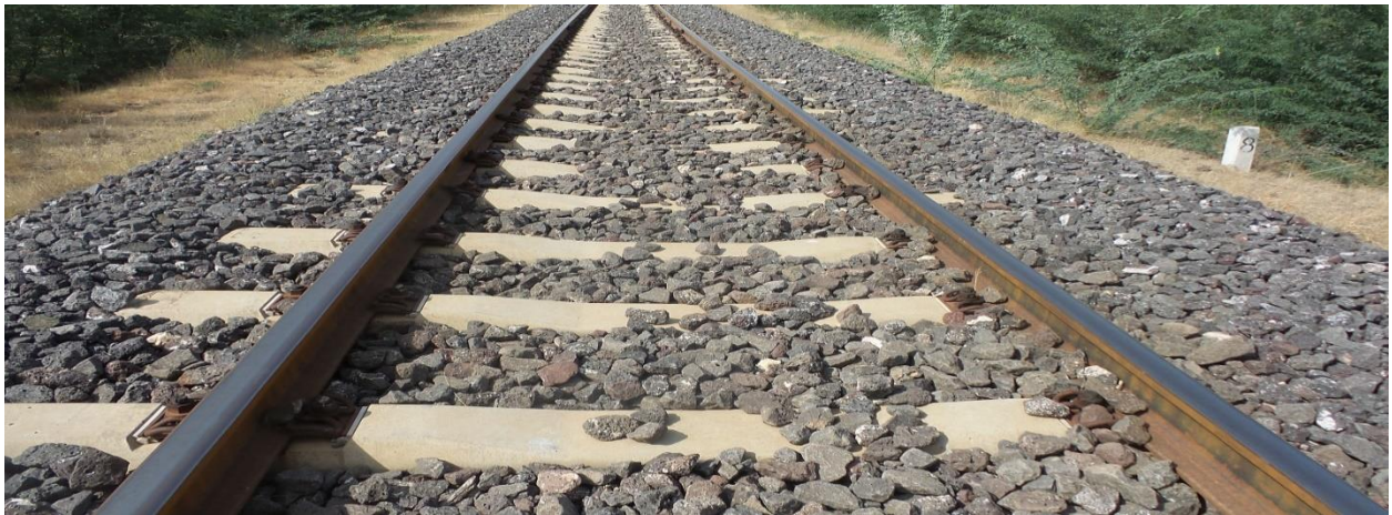
Figure 12: Cobble on main track at K470+300
