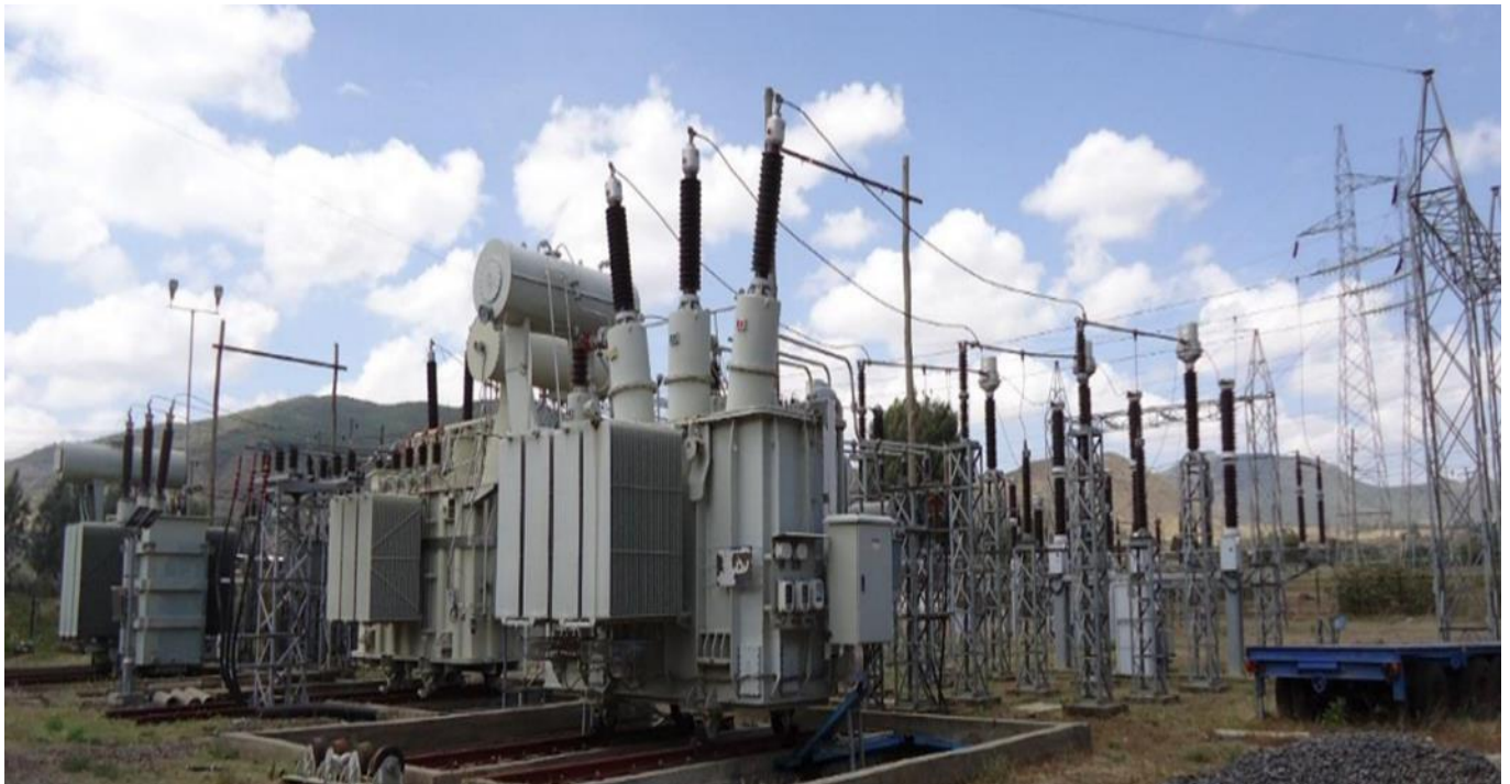
Figure 1.1 Overview of Bishoftu substation II
