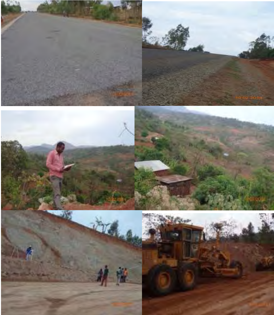
Portion of finished road surface with double surface treatment and memory of the topography of the area
