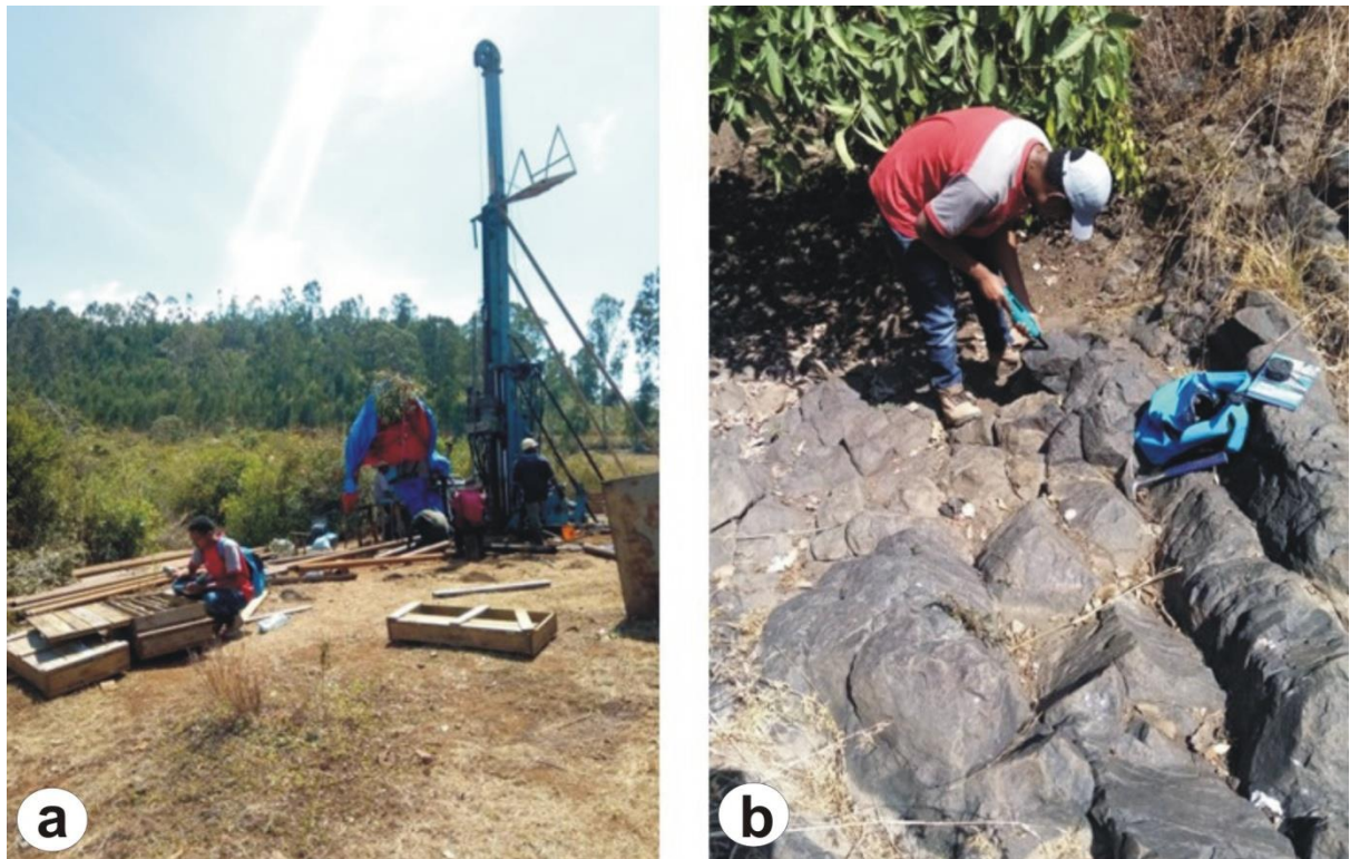
Plate 4.1 (a) Bore hole logging during field work and (b) Field compressive strength estimation using Schmidt hammer
