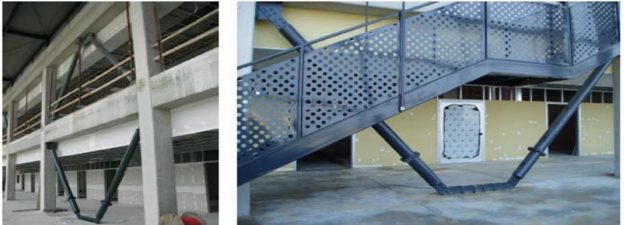
Figure 2.31. Two BRADs installed in the new building of the University of Ancona (Antonucci et al. 2006).
