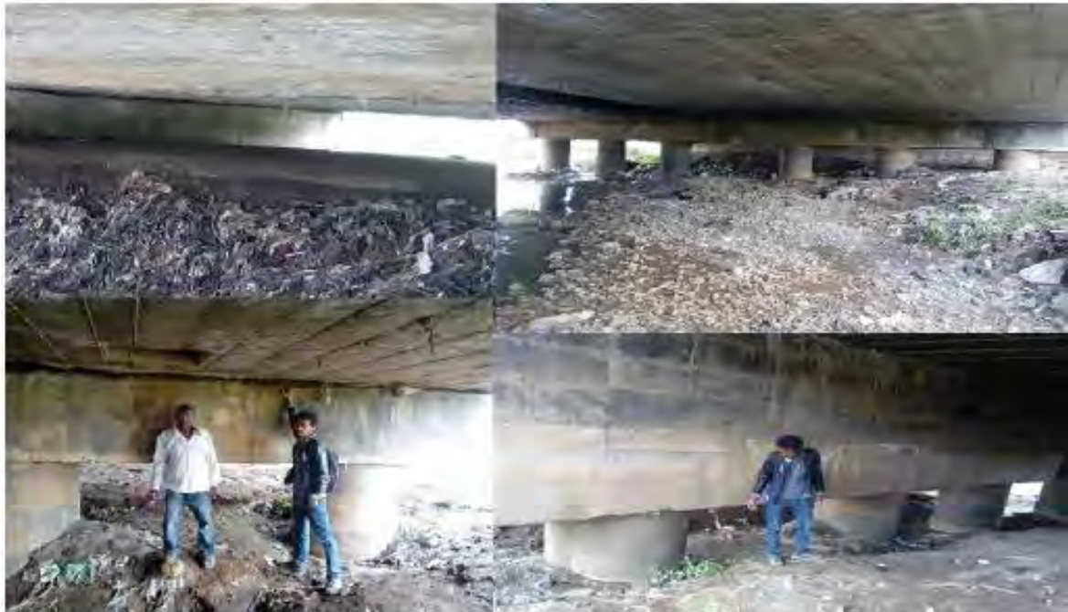
Figure 7. Current sedimentation level and Bridge condition (August 2015)
