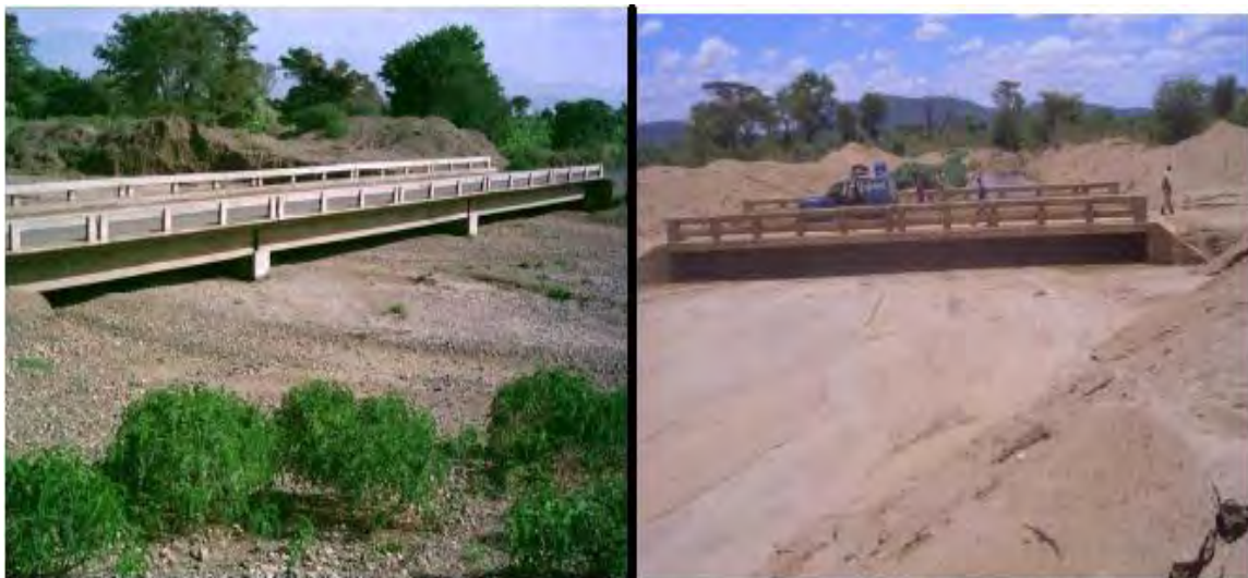
Figure 13(a) Sediment Aggradation on Segen Bridge (Right) and Baso Bridge (Left) with inadequate opening size. (Source: Beza Nigussie, 2010).
