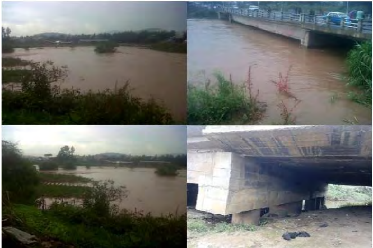
Figure 8. Flood at Mekanisa Bridge on August 2015
