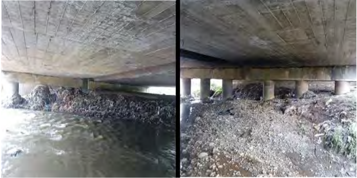
Figure 15. Debris and Sediment accumulation on piers at Mekanisa Bridge
