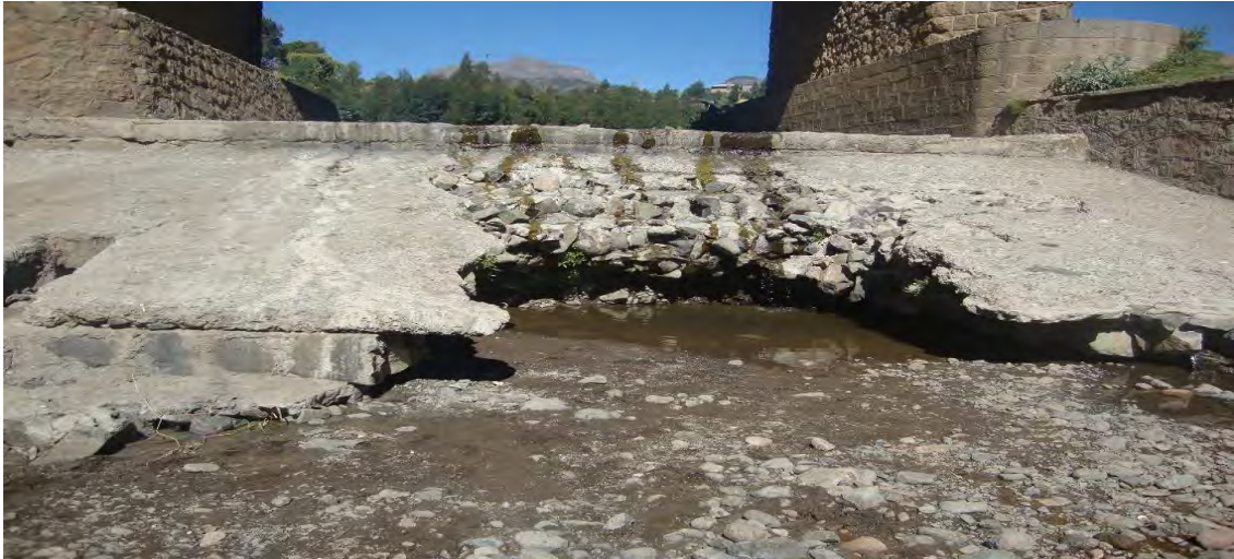
Figure 14. Pier and Foundation scour of a Bridge. (Source ERA)
