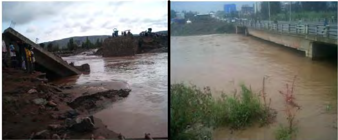
Figure 13(c). Faheem River Bridge failure due to flooding (Left) and flooding at Mekanisa Bridge on Little Akaki River due to narrowing of opening (Right). Source (Beza Nigussie, 2010) and Field visit.
