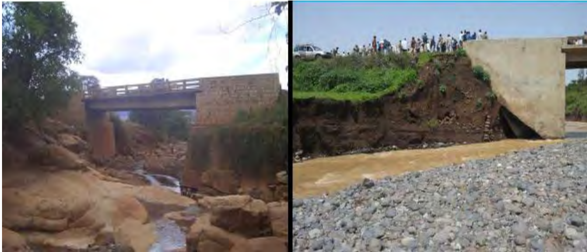
Figure 13(b). Bridge Abutment scouring on river Warda (Left) and Garno Bridge (Right). Source (Beza Nigussie, 2010).
