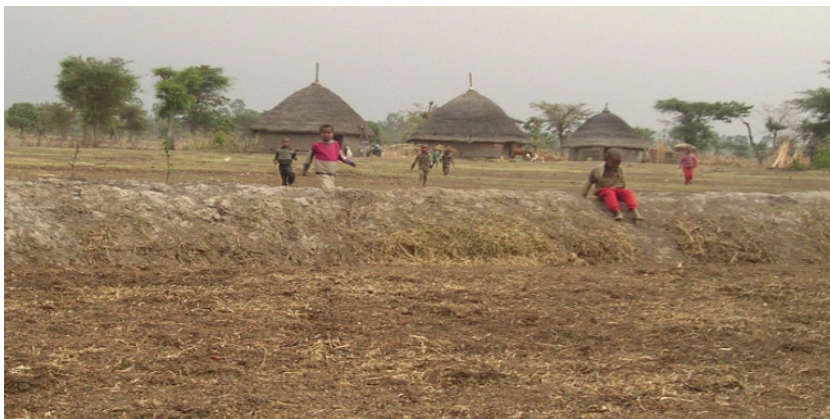
Figure 10. Flood protection structure on flat area of Shashogo, in Suta Kebele (Source, Author).
