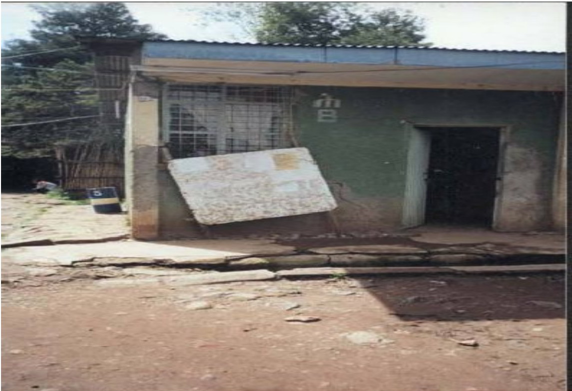
Figure 2.8 b) Detachment of tie beam and column [31]
