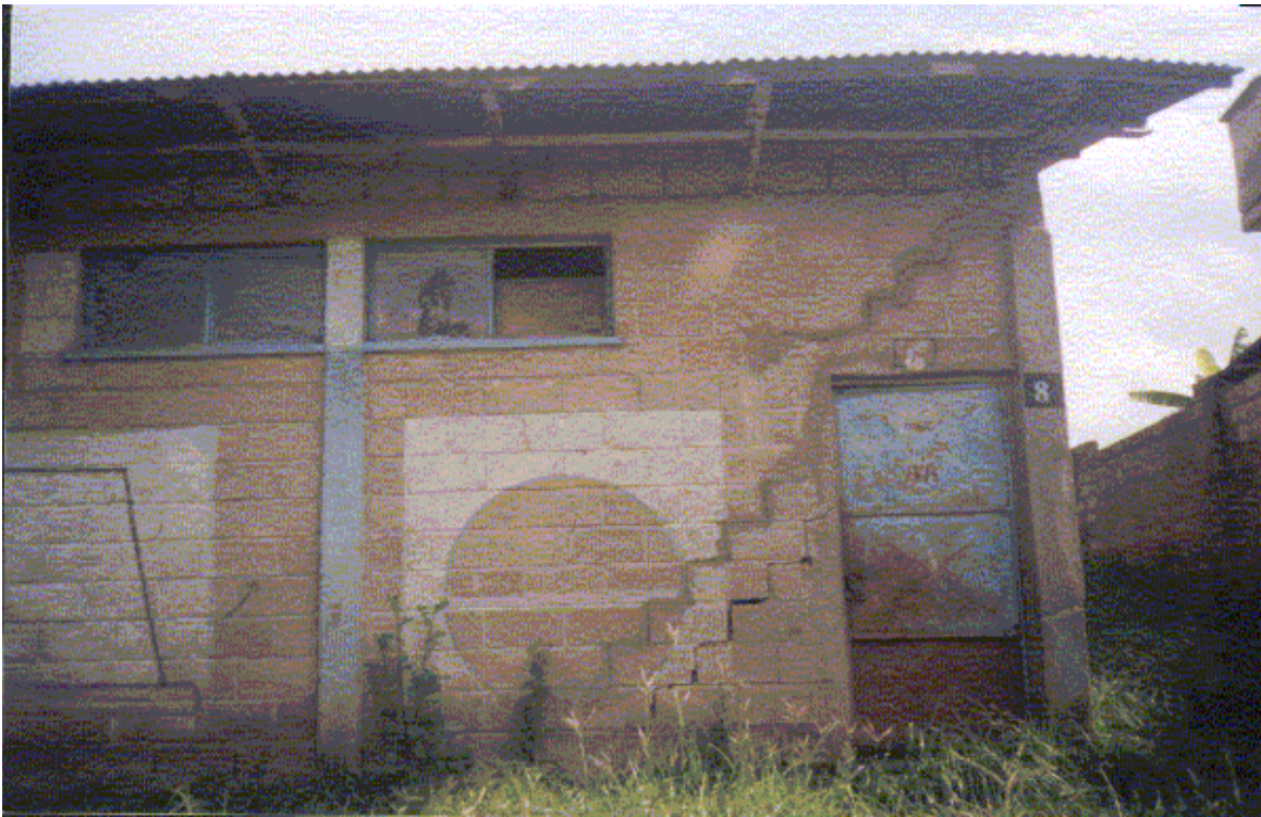
Figure 2.8 d) Sever diagonal cracks on building wall [31]
