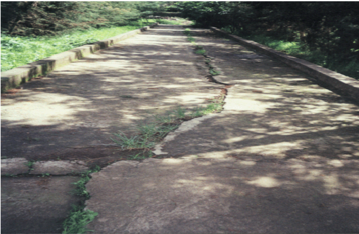
Figure 2.8 c) Cracks of walk way [31]
