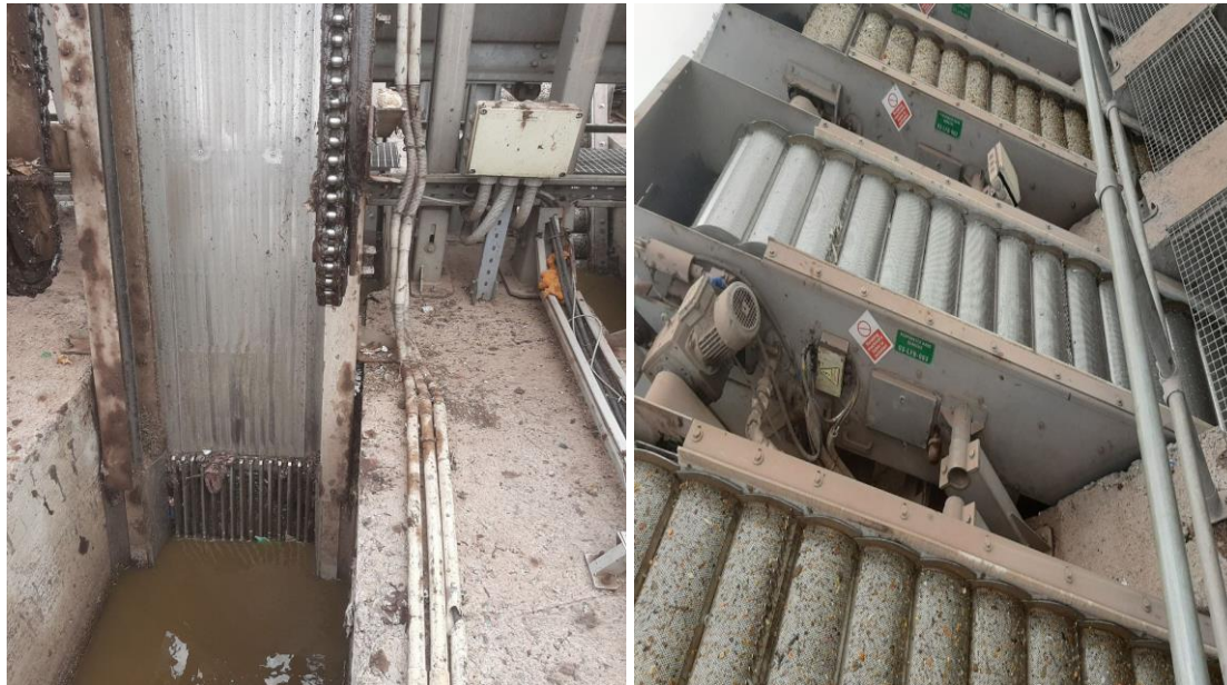
Figure 5 coarse and fine screen of preliminary treatment system
