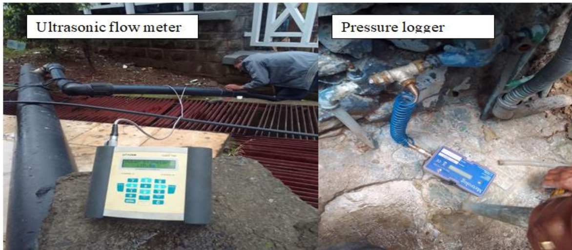
Figure 3 ultrasonic flow meter and Pressure logger
