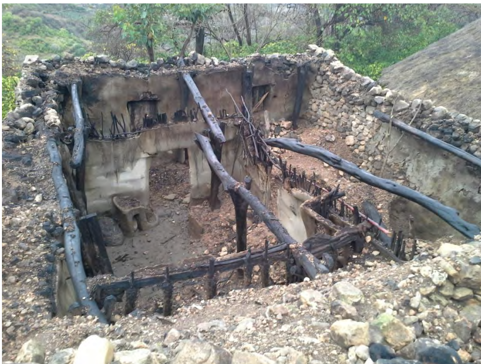
Fig. A79: Demolished house for the ned of columns & other wooden elements
