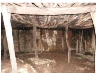
Fig.A3:6 combined space of living area and women's space due to the demolished partition
