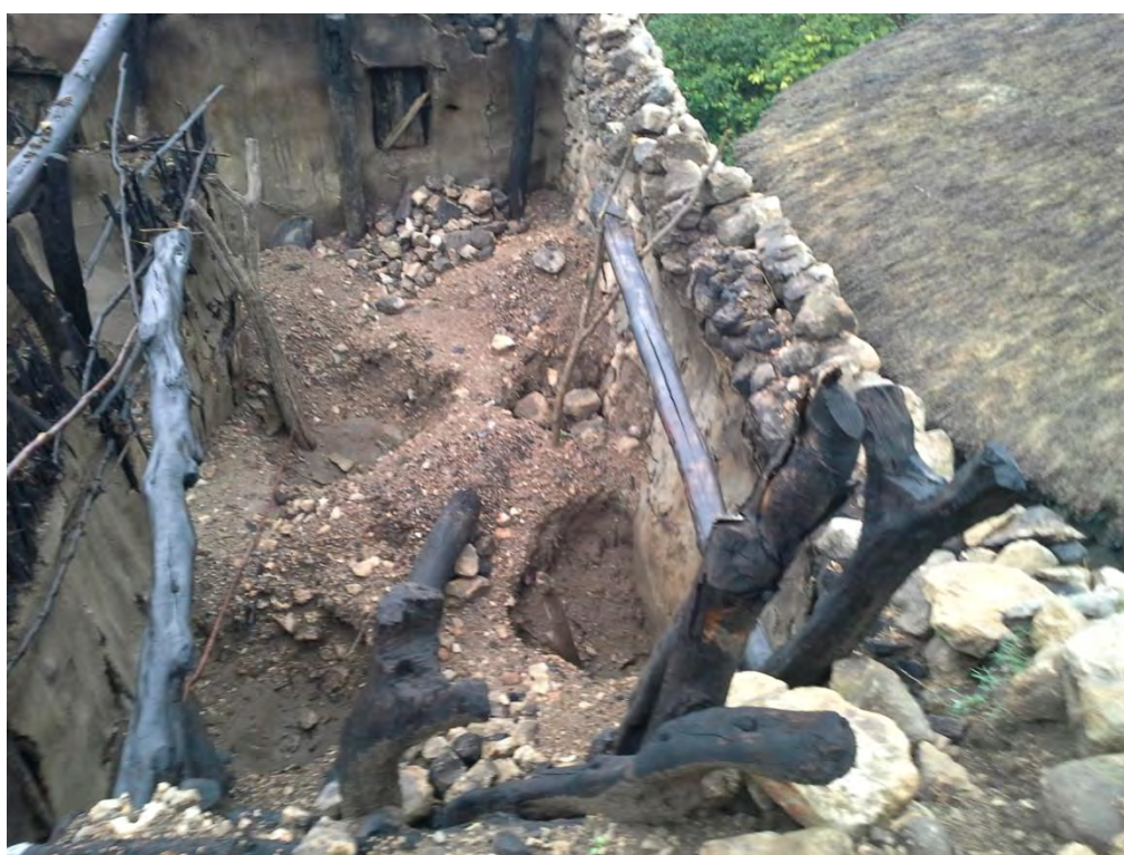
Fig. A82: Demolished for the in need of columns & other wooden elements
