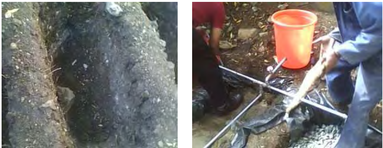
One of the microcosm cells (left) and the distribution pipe installation
