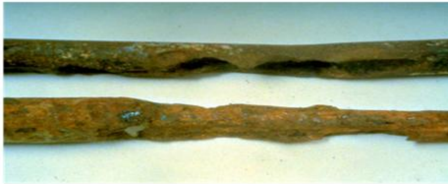
Figure 9 an example of a corrosion type called Pitting caused by chloride attack.
