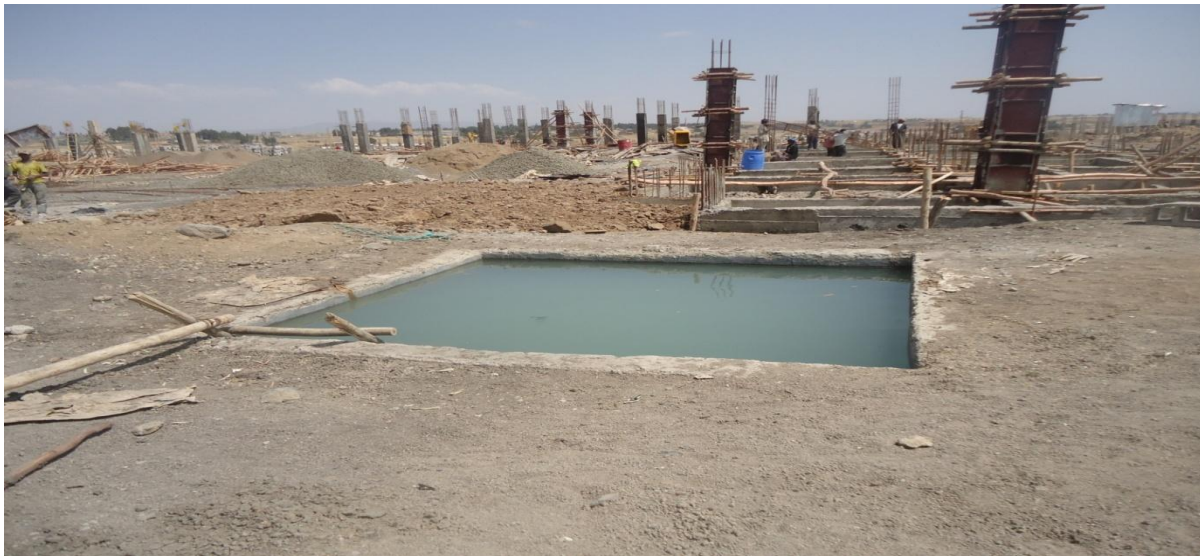
Figure 4.5 water tanks in Bole Arabsa site
