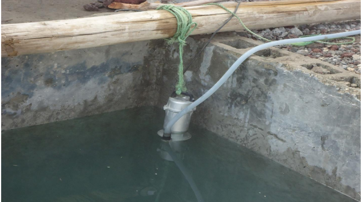
Fig 4.19 water tank in Bole Arabsa site
