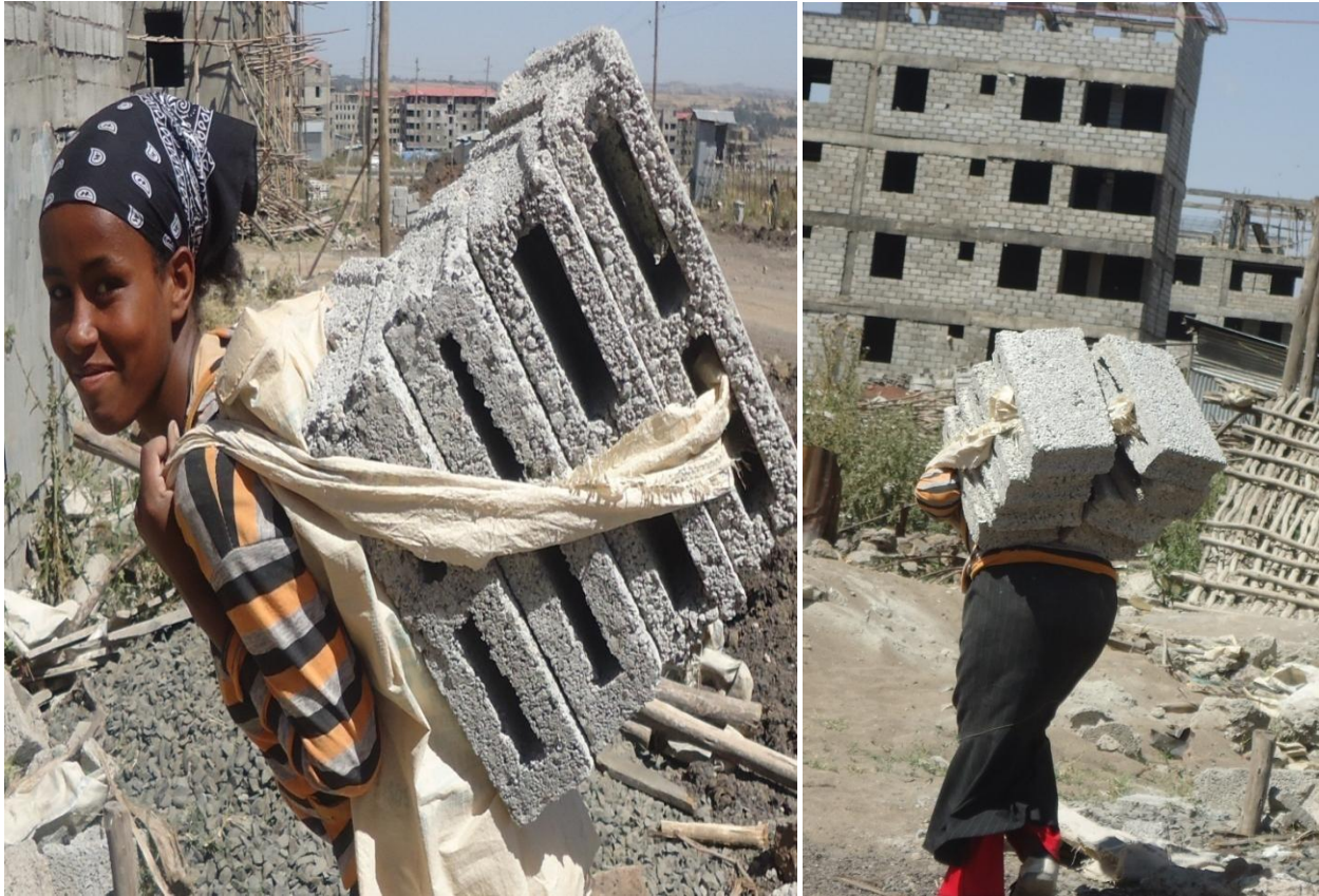
Fig 4.22 Transportation of HCB from ground to 4th floor in Yeka Ayat II site
