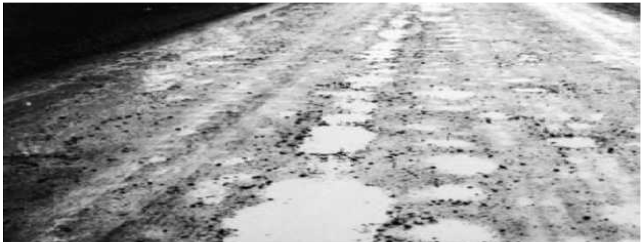
Figure 2.2: Potholes filled with water Source: Donald Walker [25].
