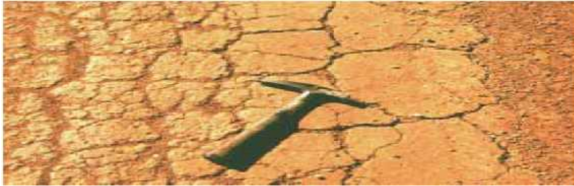
Figure 2.10: Severely Cracked Gravel Road Surface
