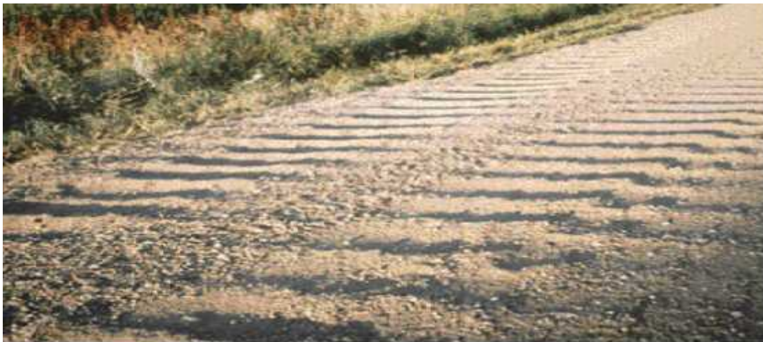
Figure2.3: Severe Corrugation Type
