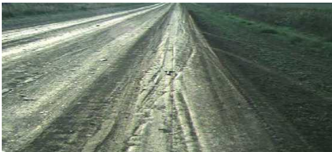
Figure 2.9: unacceptable type of slipperiness on the roads
