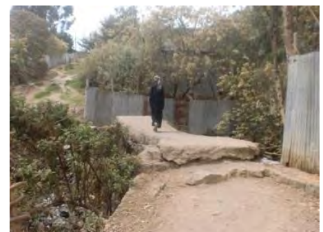
Figure 6.54: crossing the unsafe bridge
