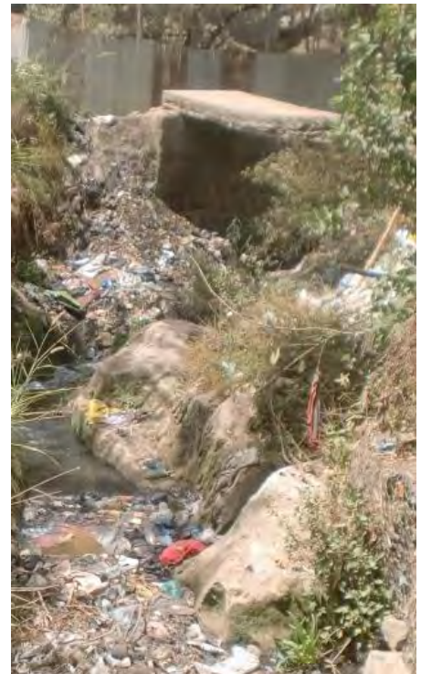
Figure 6.49: The river with waste materials
