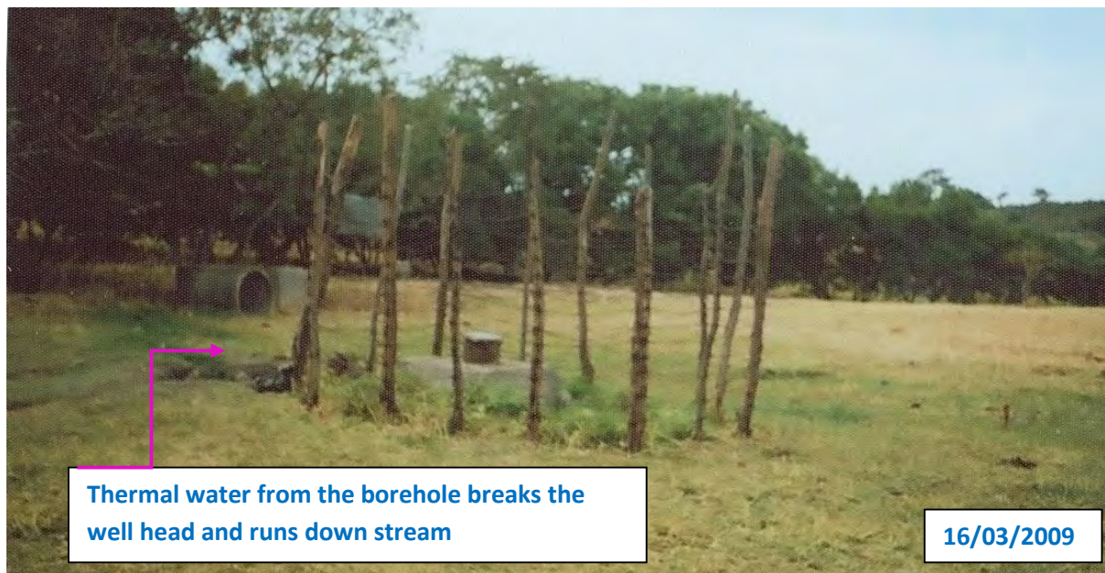
Figure 5.8 Wanzaye Borehole (thermal water)
