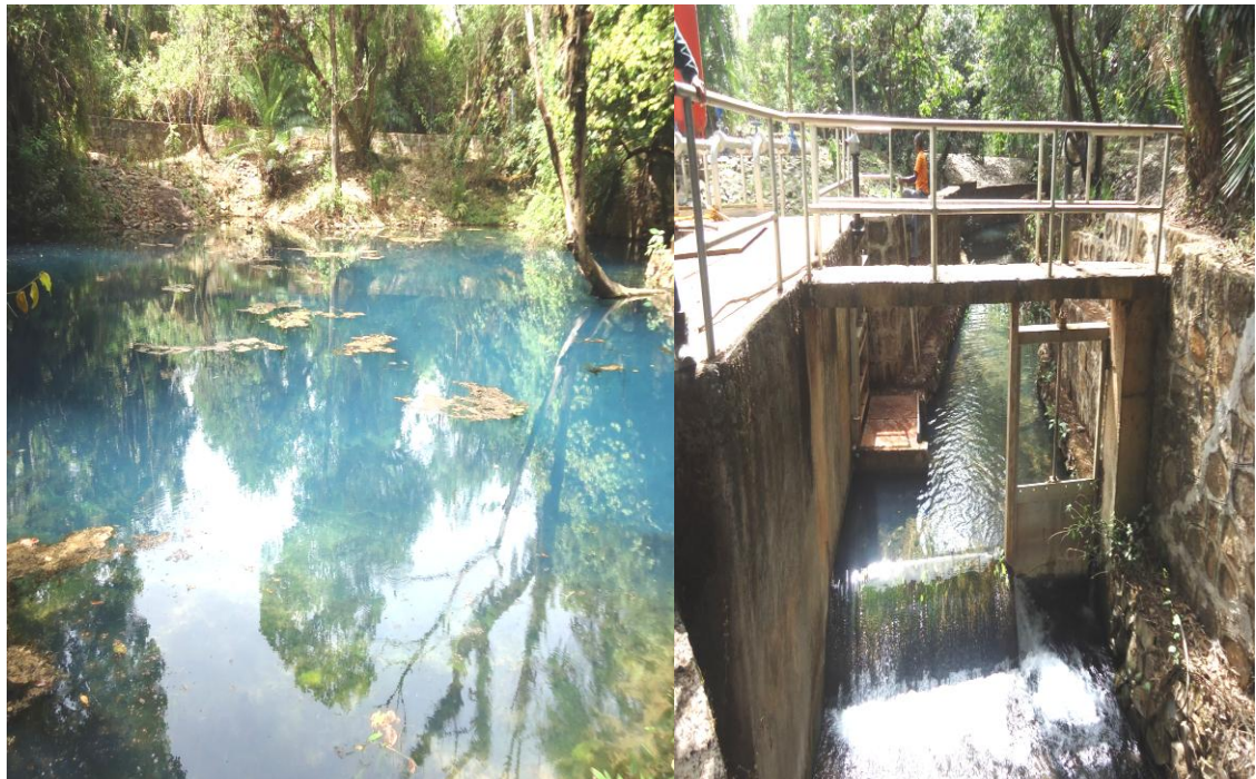
Figure 4 .Well Protected Spring Capping and diversion structure
