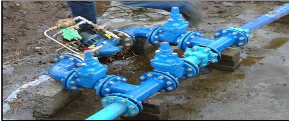
Figure.7. Typical installation of PRV
