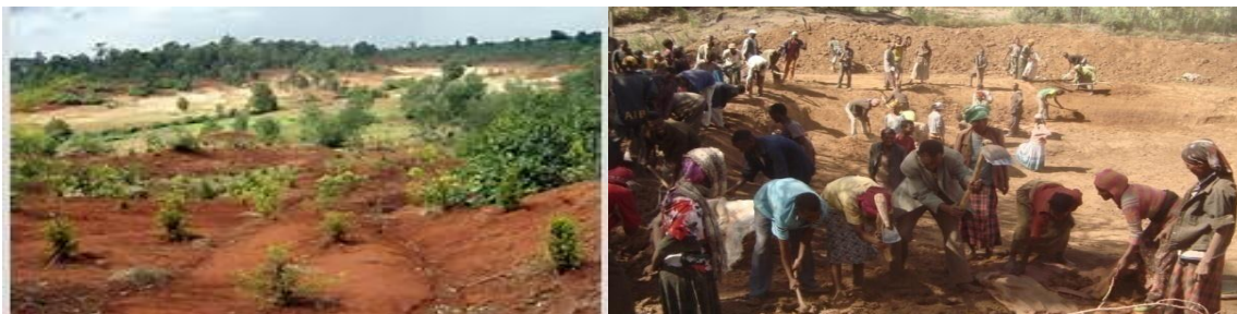
Figure 19. Closure area and water harvesting ponds in the study area public work participant farmers in bade mera village.
