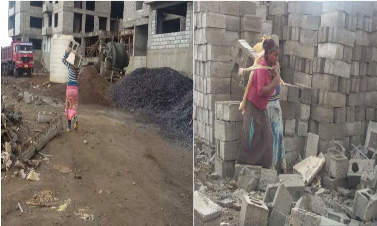
Figure 4.12 Improper handling of HCB
