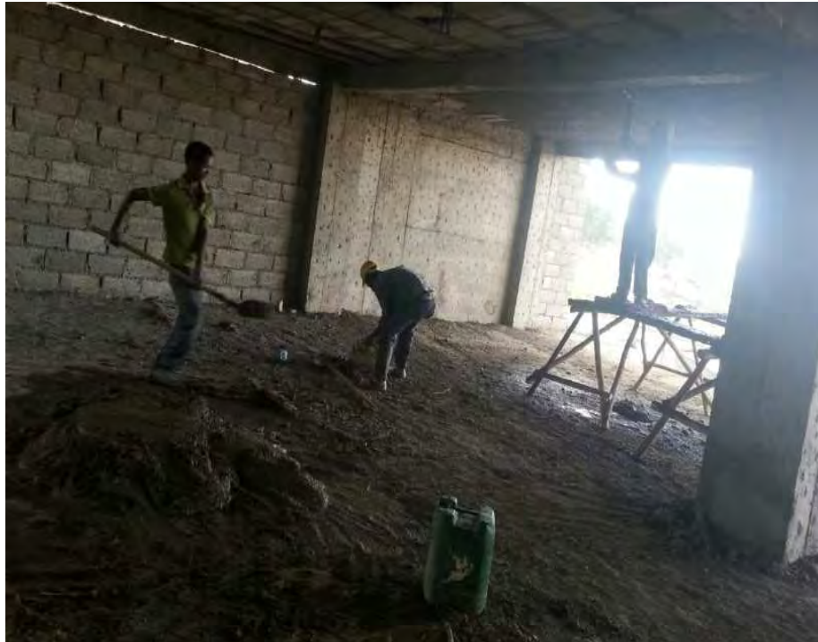
Figure 4.8 Inappropriate ways of transporting mortar
