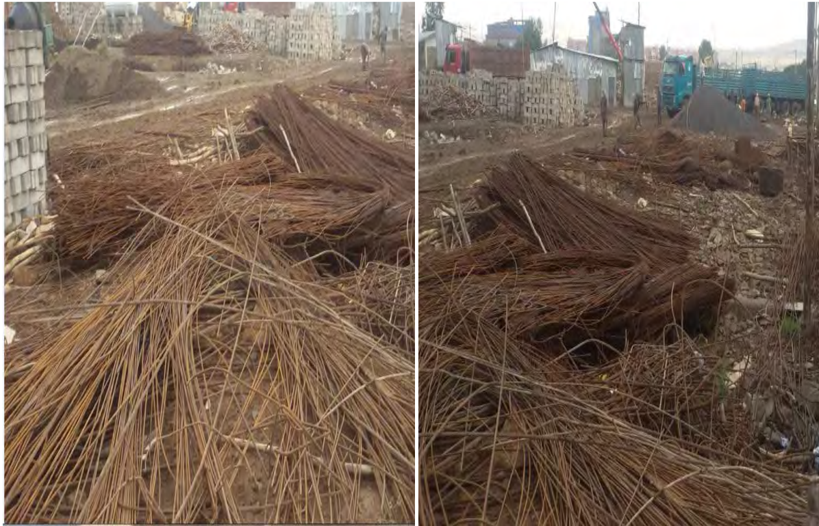
Figure 4.10 Large disorganized stocks of reinforcement bar
