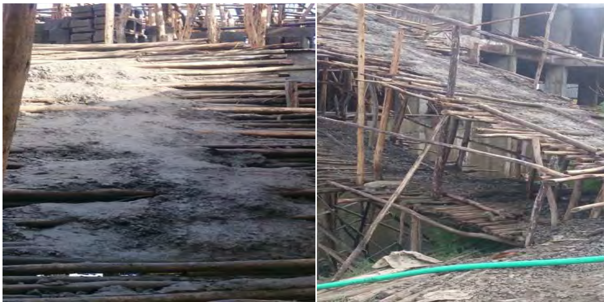
Figure 4.5 Result of improper way of transporting concrete
